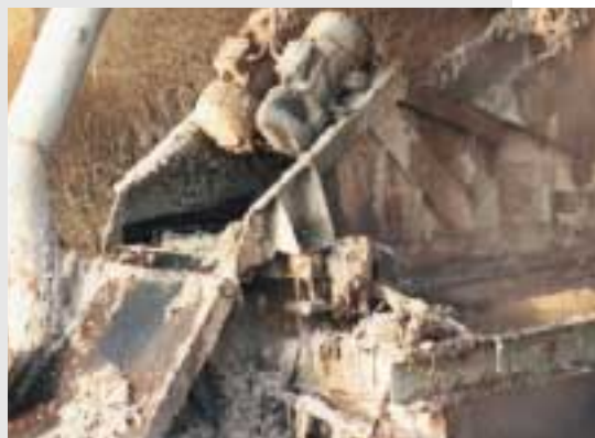
Extreme environmental conditions in paper recycling place high demands on the sealing of housings
